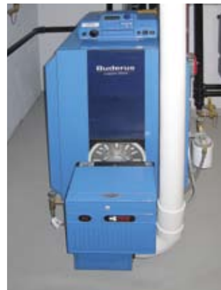
Combustion air reaches the Riello burner through a custom transition box.
