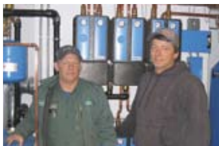
Bill Lacey (left) and Ed Dullea performed most of the installation work.
