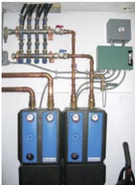
Mixing stations in the garage temper water for a radiant floor zone and the snow-melt system.
