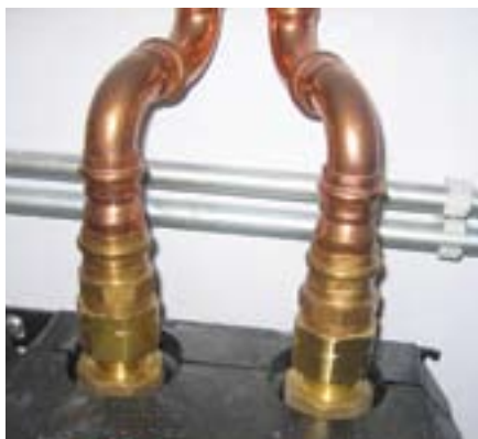
Joints on the pumping stations were made without solder using the Viega ProPress system.
