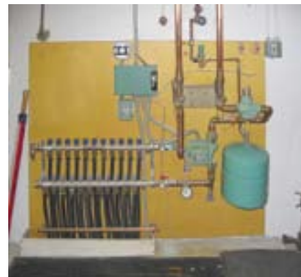
The snow-melt system features a plated heat exchanger and an expansion tank.
