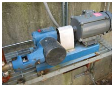
Bulk plant injection systems can treat a large volume of fuel at once, but are more costly than other methods.
